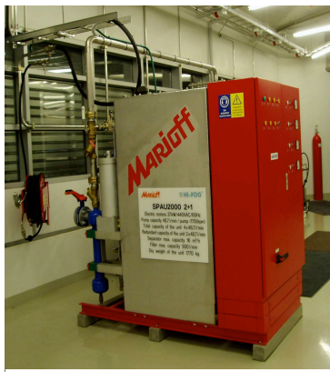
High pressure water mist pump set and control unit.
