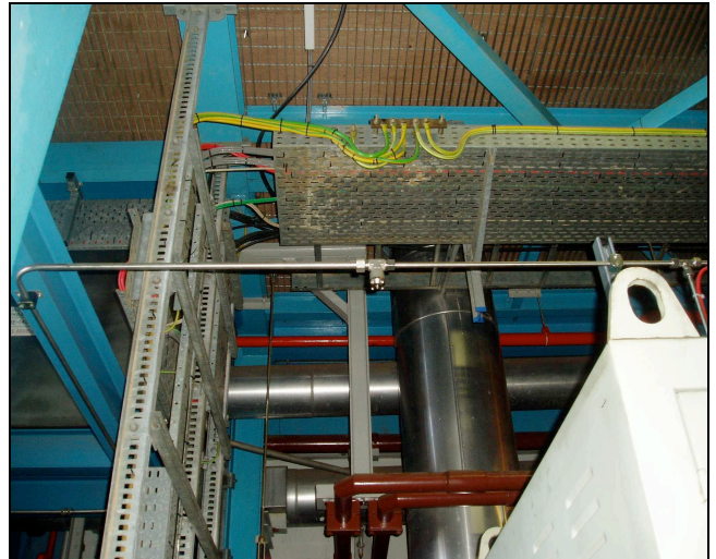
Mist nozzles and stainless steel pipework for a system in a power station
