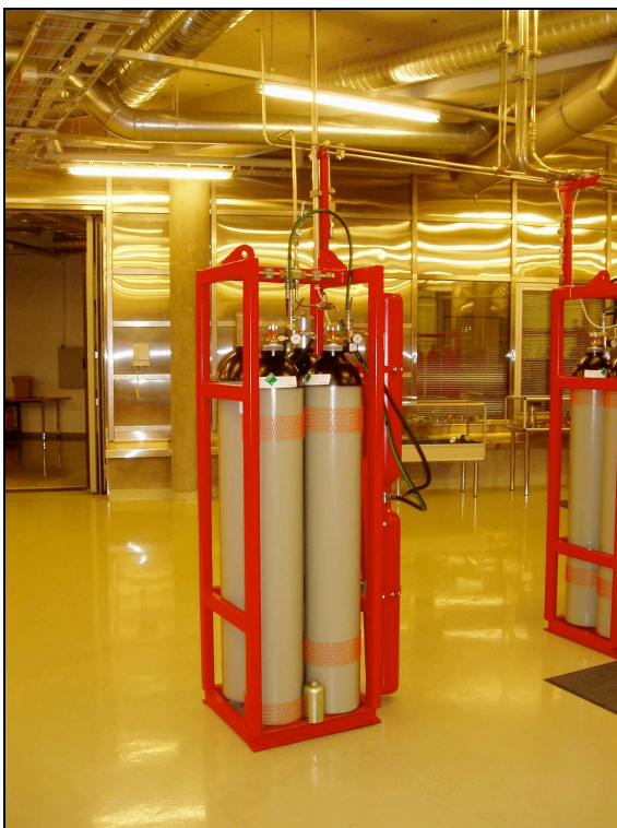
Replacement gas cylinders for a mist system
