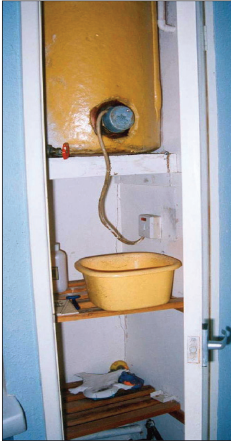
Airing cupboard with hot water tank above
